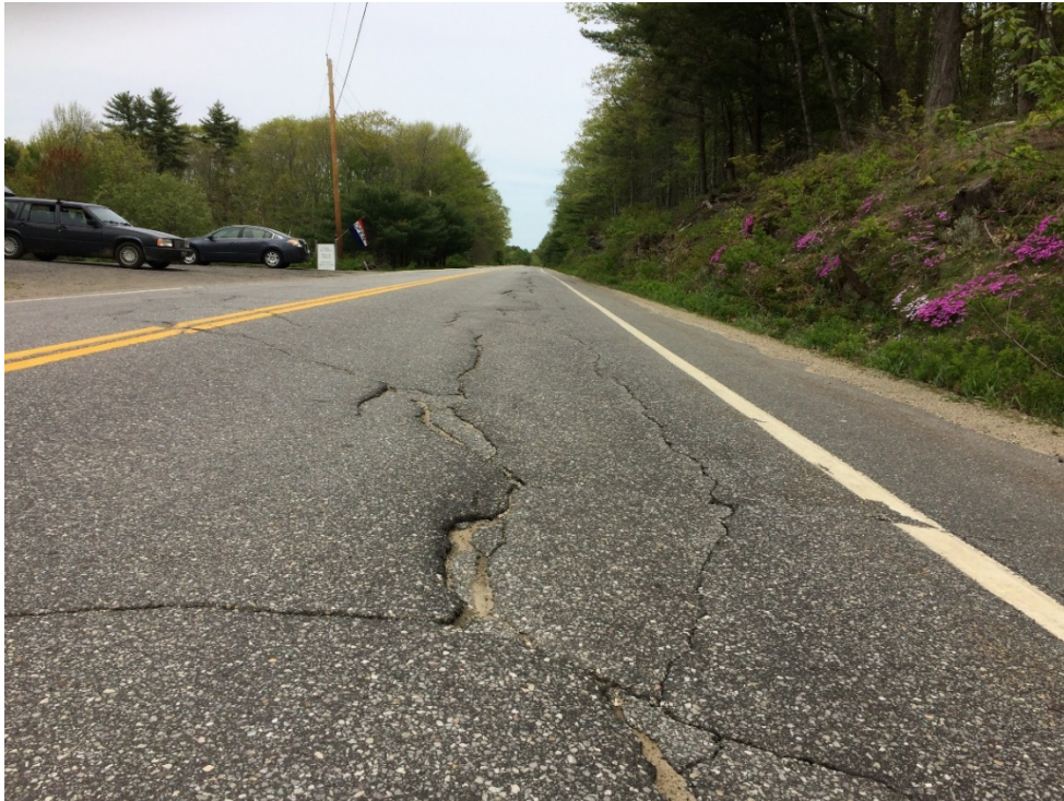
Present road conditions on Route 129 near the Walpole Meetinghouse
