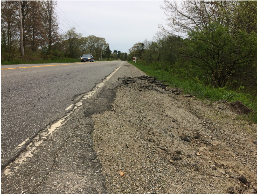
Present shoulder conditions along Route 130 south of Bristol Mills
