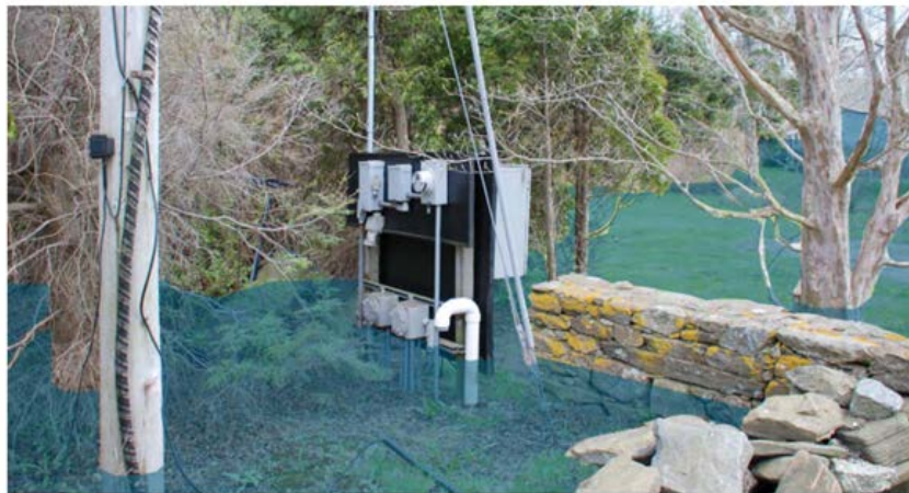
PS #12 Electrical / Controls Panel Looking South - BFE +4
